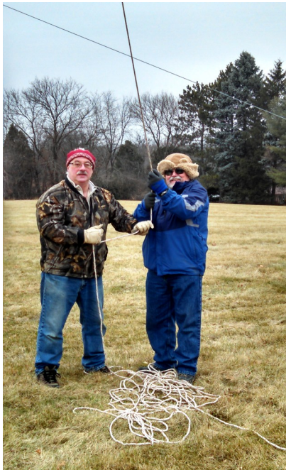
John Huntley and Kurt Eversole raise the new antenna to the tower climber.
