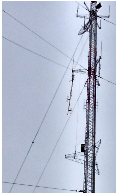
Up, up, up, to the 350' level on the tower that our antenna is positioned.
