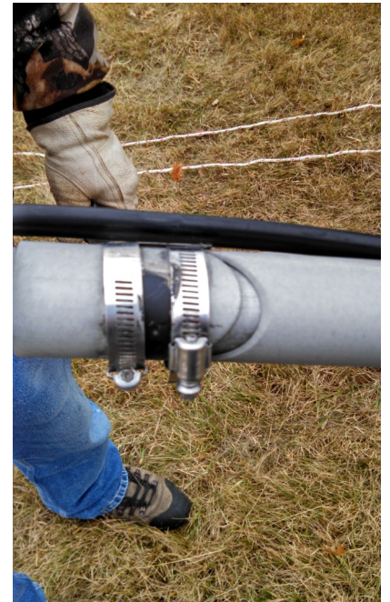
Inspection of the old antenna shows the possible failure point that would have occurred in time.
